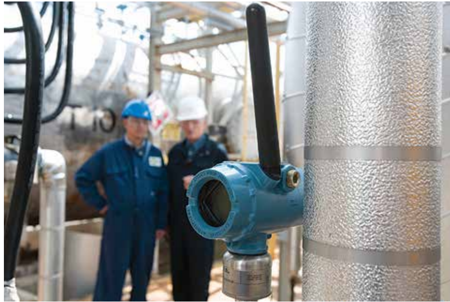
FIG. 1. A WirelessHART project typically involves the end user, the wireless equipment vendor and perhaps a systems integrator.
