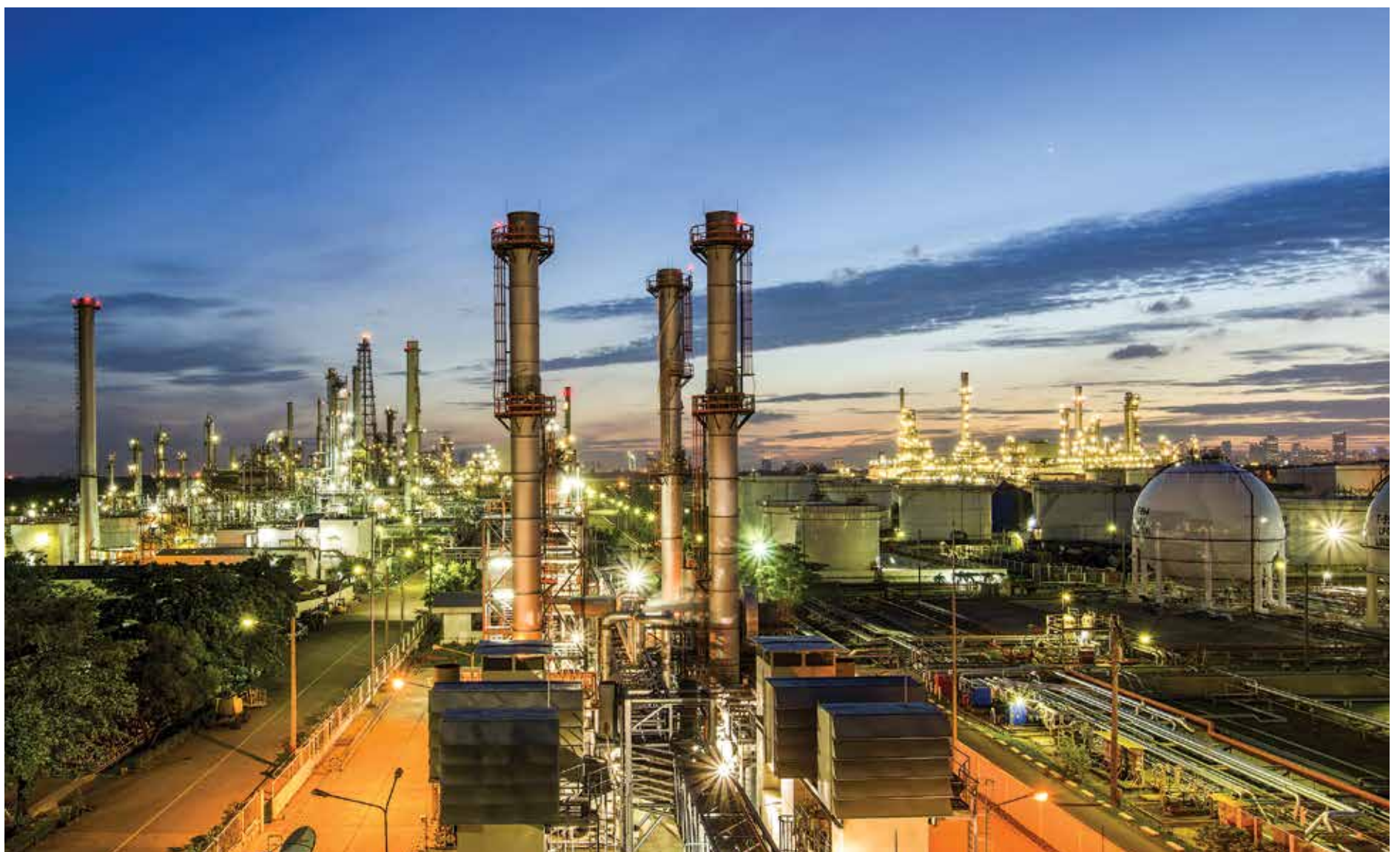
FIG. 1. Best-in-class planning and scheduling technologies improve visibility across the entire petroleum supply chain and increase profitability.
