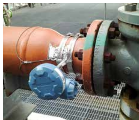
FIG. 2. A WirelessHART acoustic transmitter clamped to a pipe.
