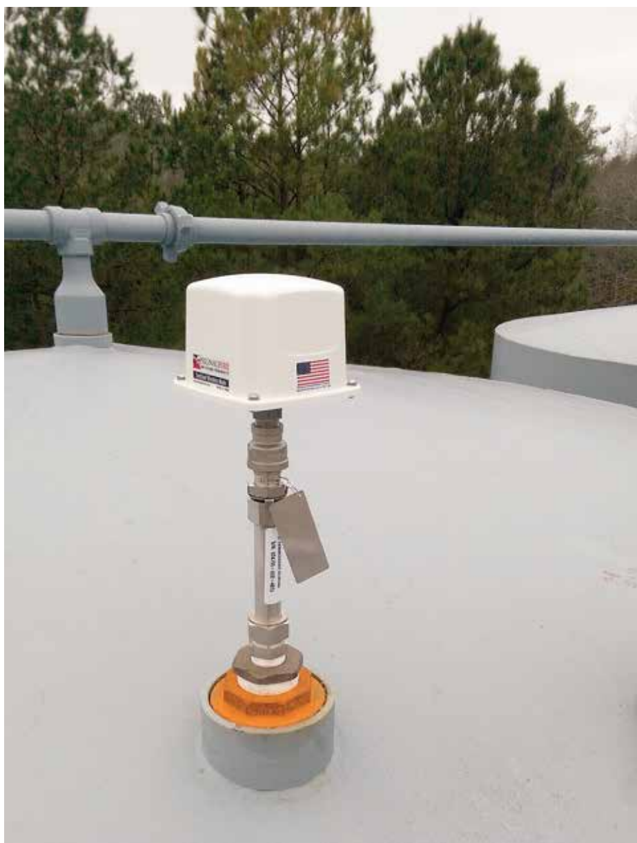
FIG. 1. To provide wireless tank level monitoring, the SignalFire Remote Sensing System uses low-cost, medium-range C1D1-certified nodes that interface with sensors to provide robust, reliable wireless mesh data transmission in rugged outdoor environments.
