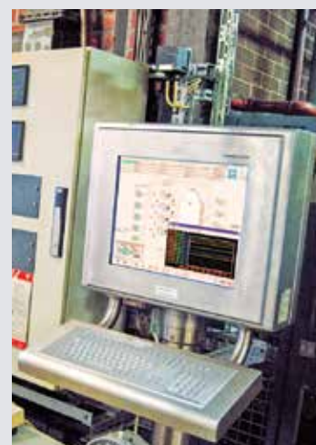
Pepperl + Fuchs details the consolidation of systems into a central, virtual machine
