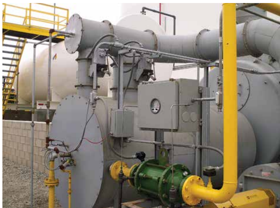
FIG. 1. S&SE's VRU&D Systems manages VOC recovery and destruction by incorporating oxidizers directly in the VRU system.
