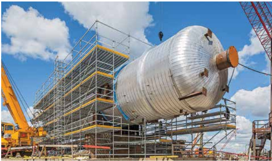
FIG. 1. The North West Redwater Sturgeon Refinery Project in Canada utilizes the integrated scaffolding solution. Scaffolding is placed around the vessel for insulation, painting and fireproofing activities.
