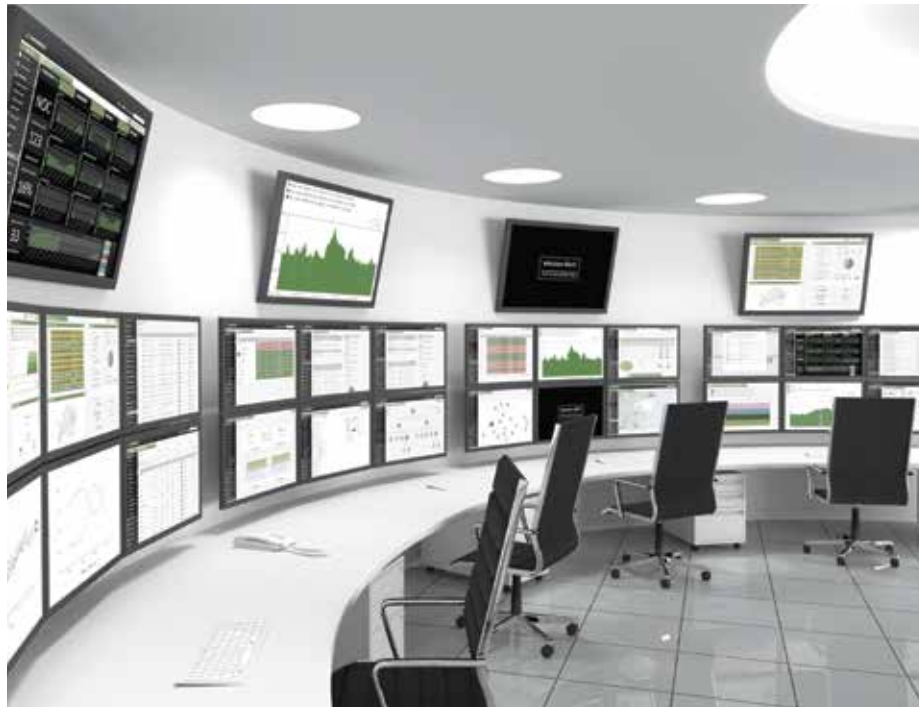
FIG. 1. Real-time alerts can enable quick identification of potential problems, allowing engineers to prevent disruptions caused by unauthorized changes to critical controllers.
